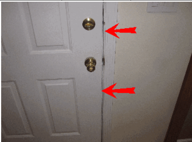
Front door weather stripping is open.
