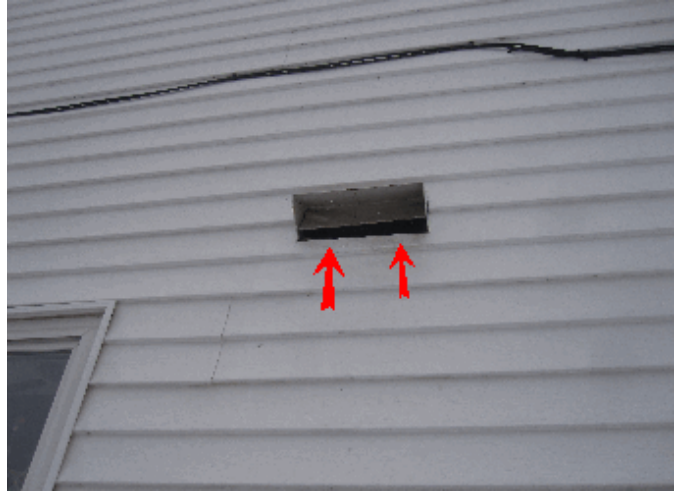
Exterior: Vent on exterior is ????. Needs to be sealed to prevent critters from entering house.
