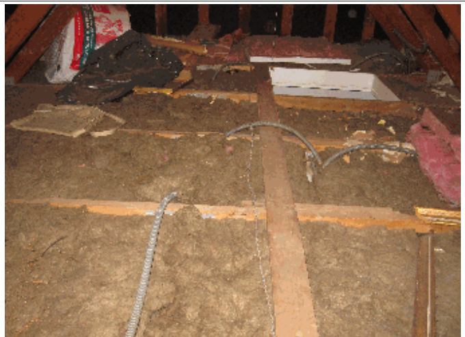
Inter: Bad attic insulation, compressed, damaged or missing.
