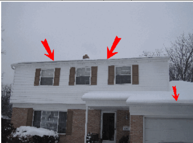
Gutters are sagging. Need to be leveled to prevent water from running over onto foundation.
