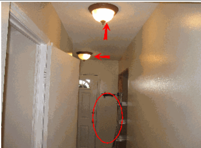
Elect.: Make sure to use appropriate dimmable bulbs for any dimmable switch light.
