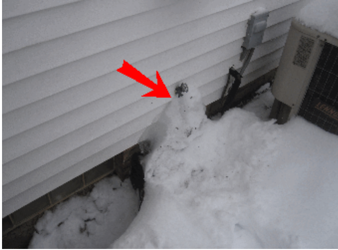
Exterior: Spigot is leaking and freezing. Replace with freeze proof spigot.
