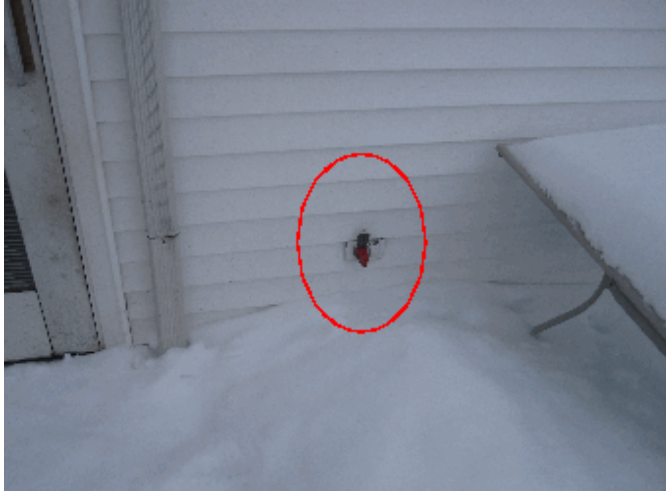
Elect.: Need GFCi outlet on exterior.
