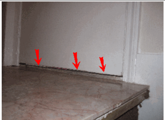
Garage entry door weather stripping is missing.
