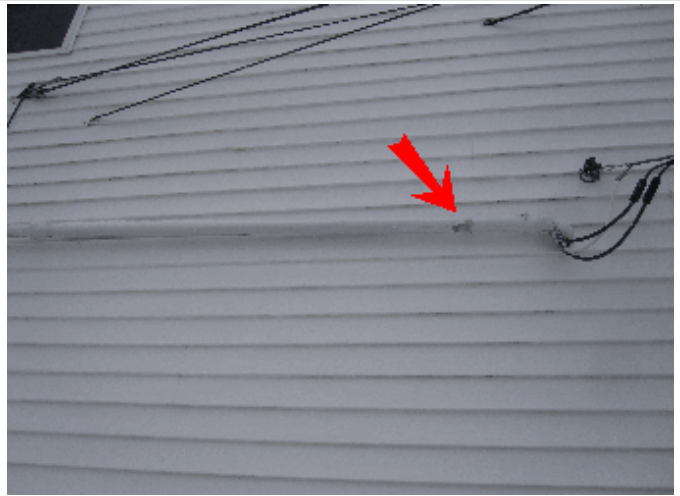
Main electrical mast needs secured to house.
