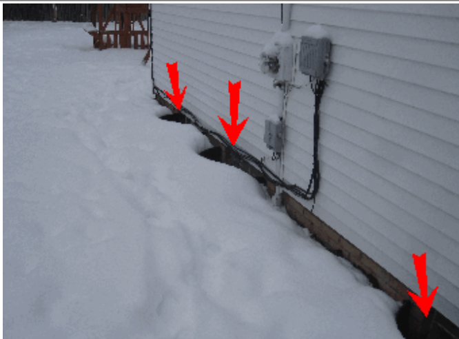
Exterior: Recommend window well covers for basement windows.
