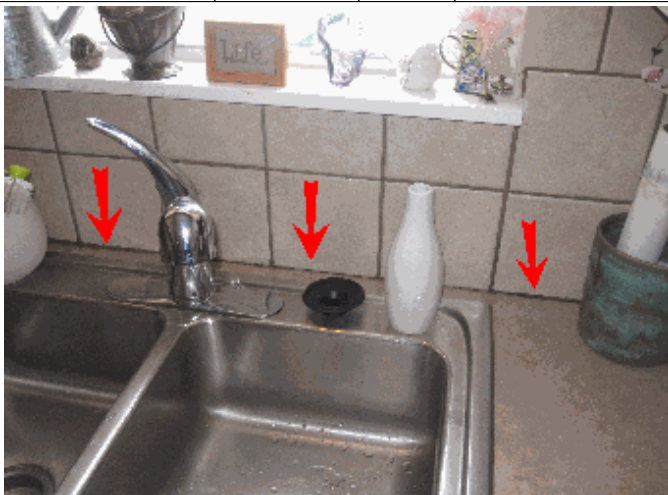
Caulk around kitchen backsplash. Open gap needs to be sealed.
