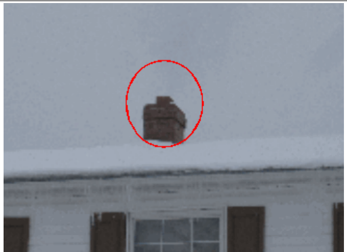
Rain cap/Spark arrestor is needed on BOTH chimneys.
