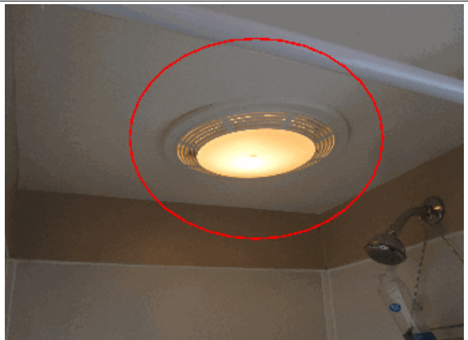
Both upstairs bath vents are noisy.
