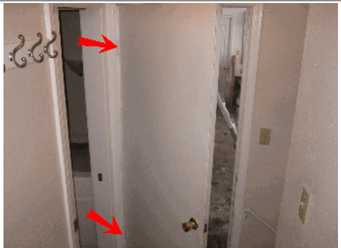
Kitchen garage entry door needs to be an auto- closure for safety/fire hazard.
